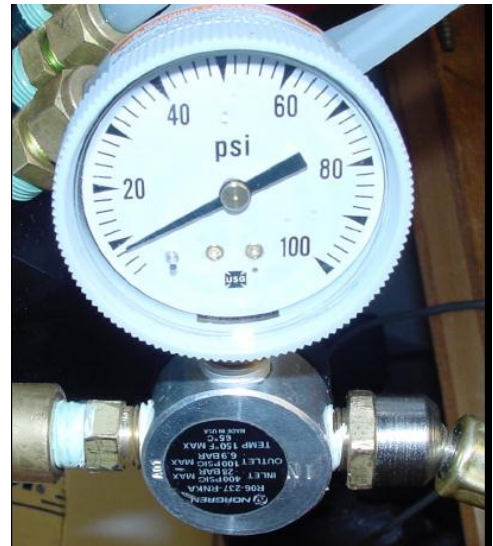
Figure 4: Pressure Gauge Showing the Inlet Pressure
